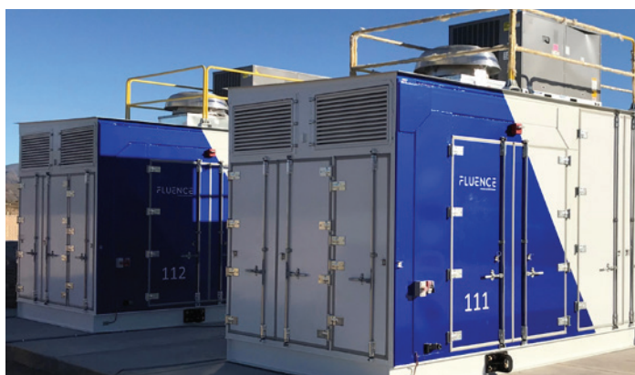
Arizona Public Service, a 2 MW, 4-hour duration system that will take the place of rebuilding about 20 miles of transmission and distribution poles and wires.
