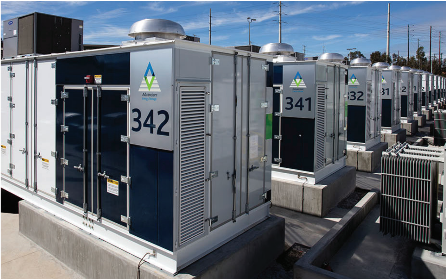
AES Energy Storage and San Diego Gas & Electric's Escondido 30 MW, 120 MWh energy storage facility in CA, one of the biggest lithium ion battery installations in the world.
